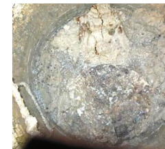
City of Phoenix Manhole Full of Grease
