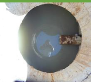
Interceptor missing outlet, no grease retention
