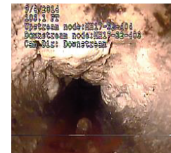
City of Phoenix Sewer Line Full of Grease
