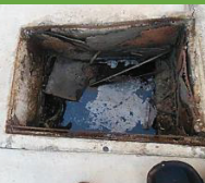
Rusted out grease trap
