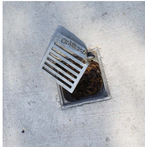
Clogged drain inlet
