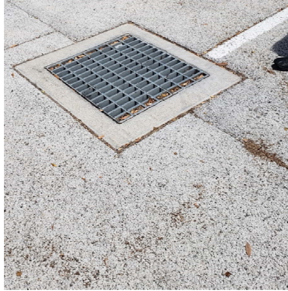
Loose leaf debris in pervious concrete
