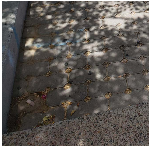
Debris on Pavers
