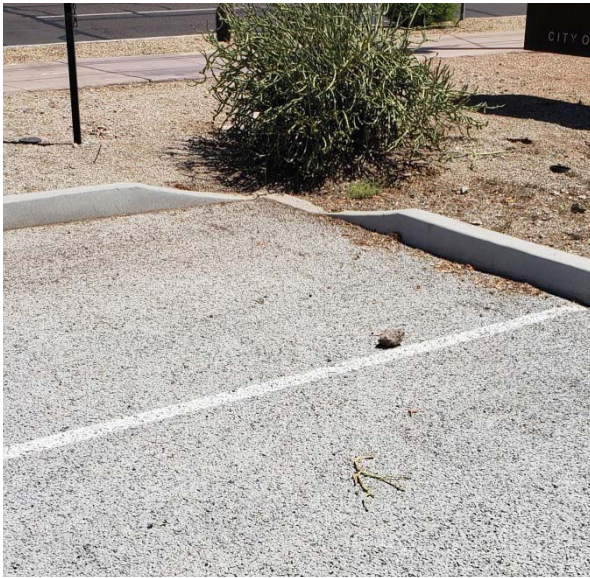
Debris buildup at sump locations
