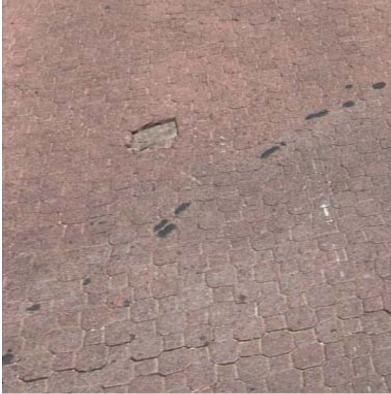
Intersection pavers missing and stained with oil and grease
