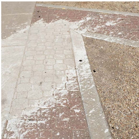
Paint spill over pavers
