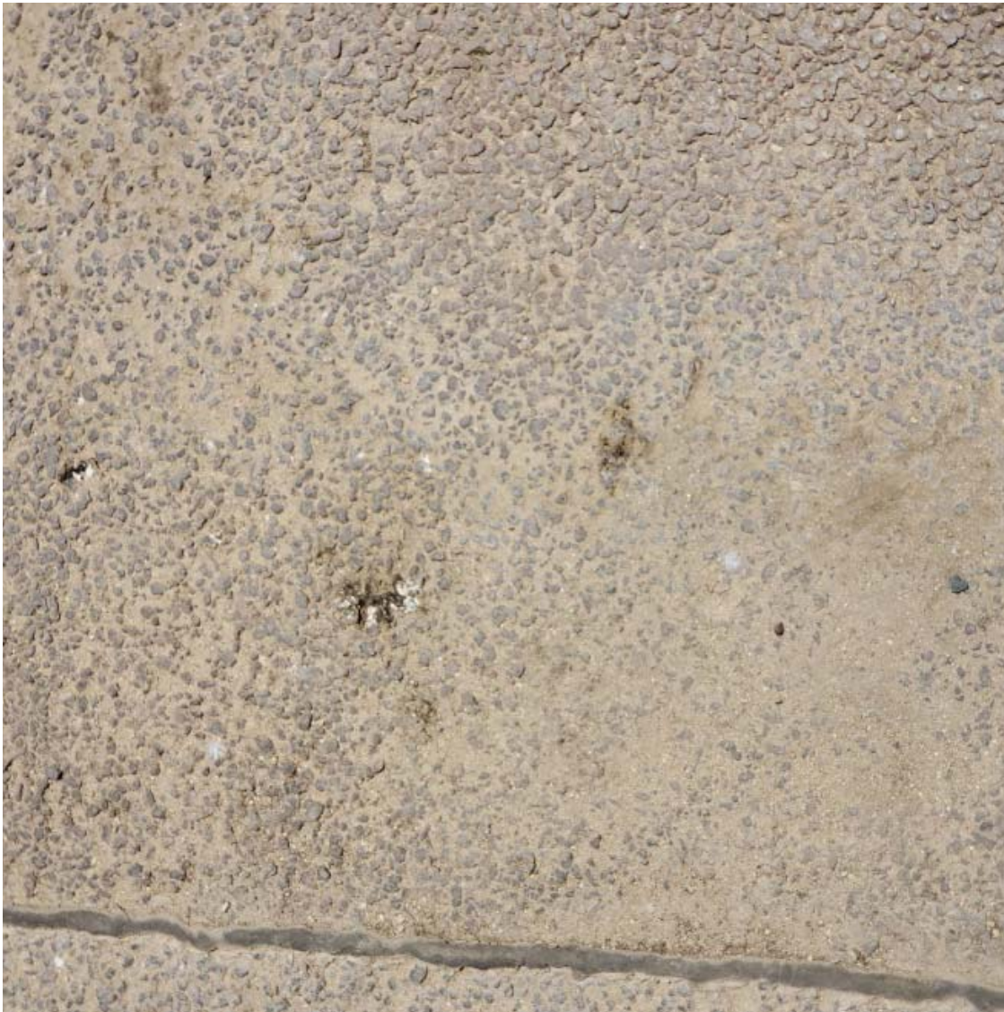
Pervious concrete full of sediment
