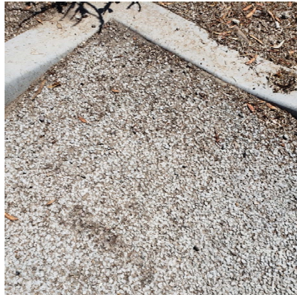
Sediment buildup at sump locations
