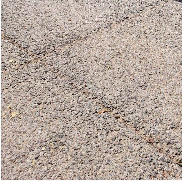
Sediment filling surface voids
