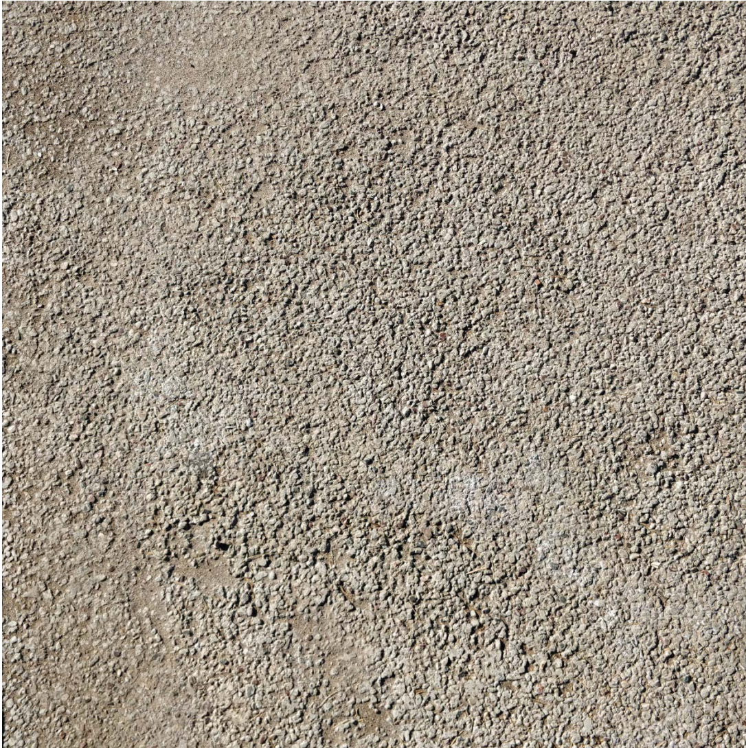
Sediment filling surface voids
