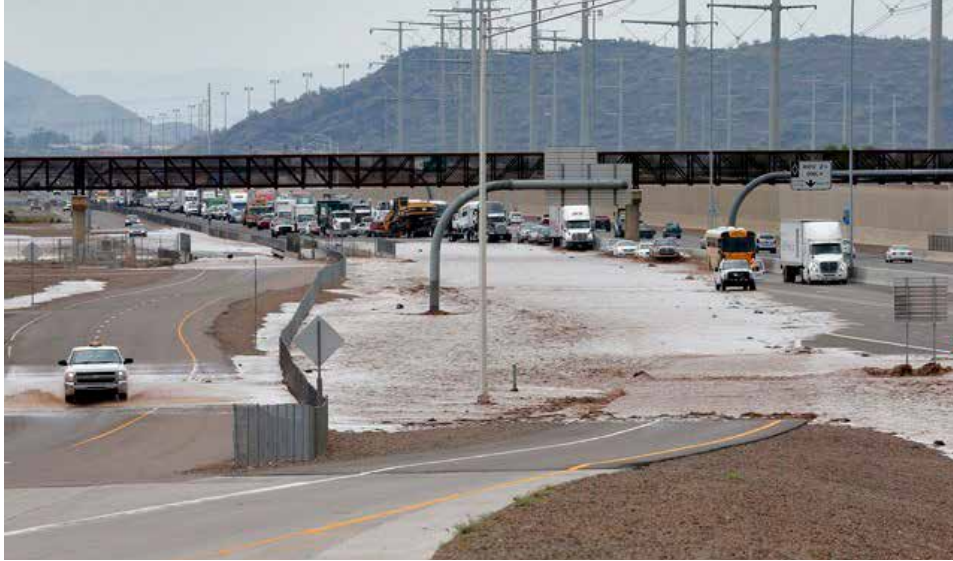
Figure 16 – Skunk Creek Overflow Floods Interstate 17, August 19, 2014
