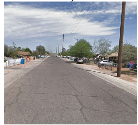
Lack of traffic calming measures to slow traffic
