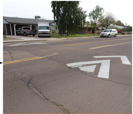
Example of speed hump
