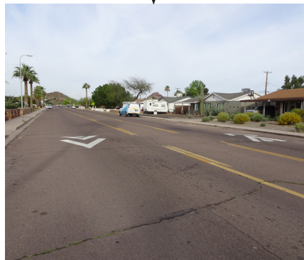
Example of speed hump
