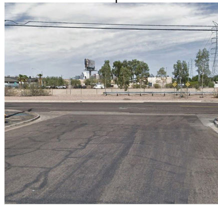
Lack of clearly marked crosswalk
