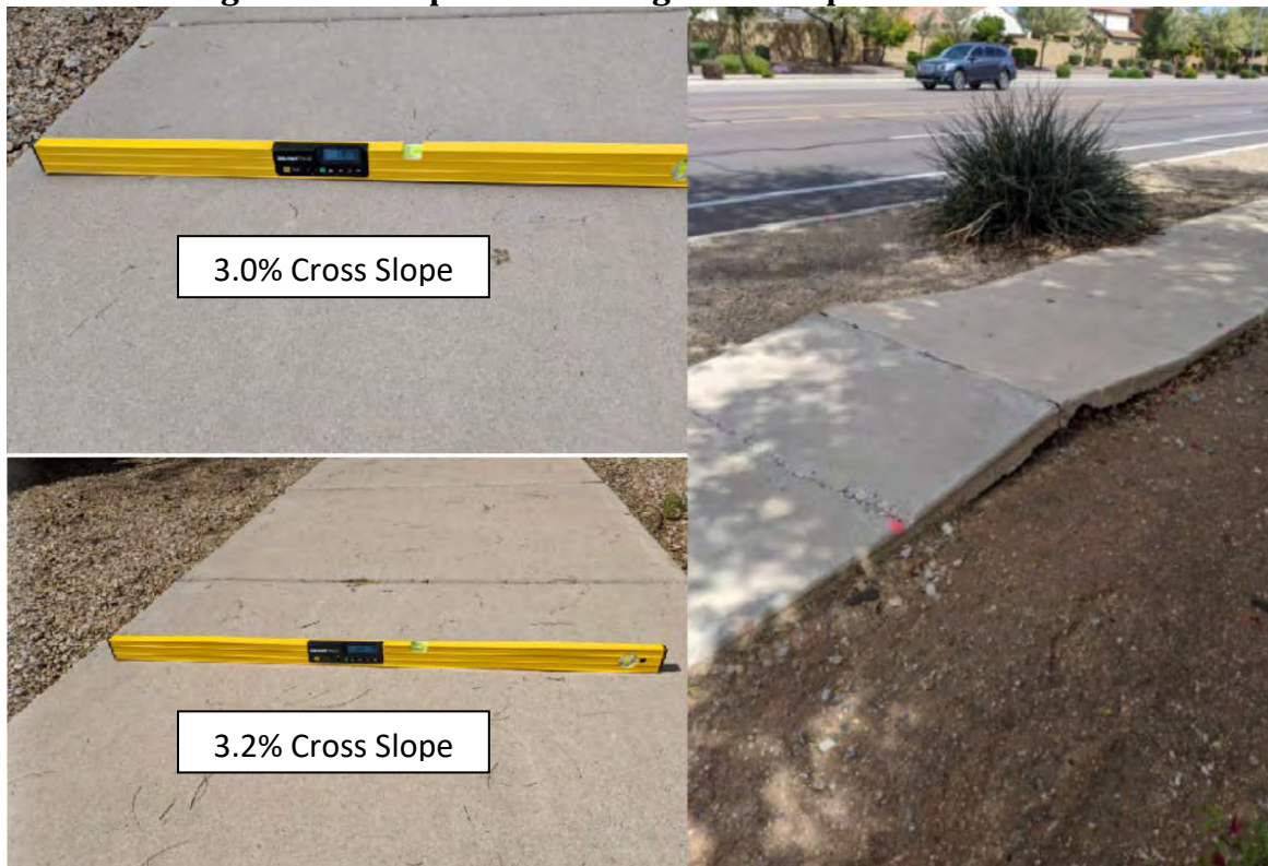
Figure 9: Examples of Existing Non-Compliant Sidewalks
