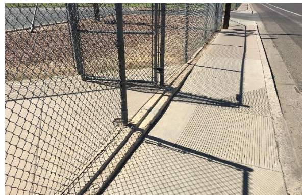
Non-standard sidewalk ramp on 39 th Ave.
