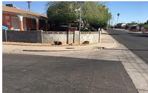
No sidewalk ramp at the corner of Verde Ln. and 44 th Ln.
