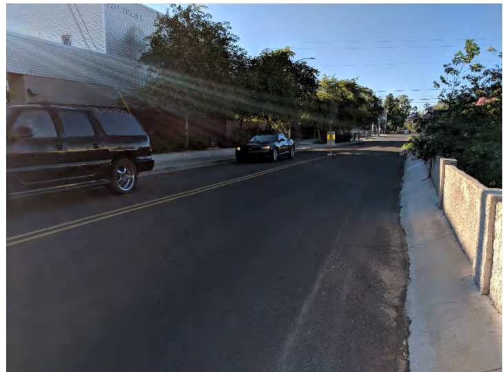
Figure 35: Sidewalk Gap on 3 rd Street south of Vogel Avenue
