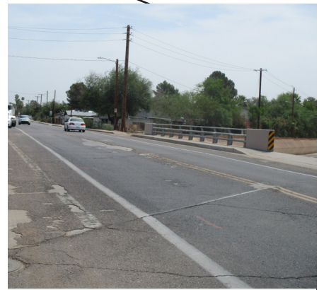
Lack of designated crosswalk at Grand Canal
