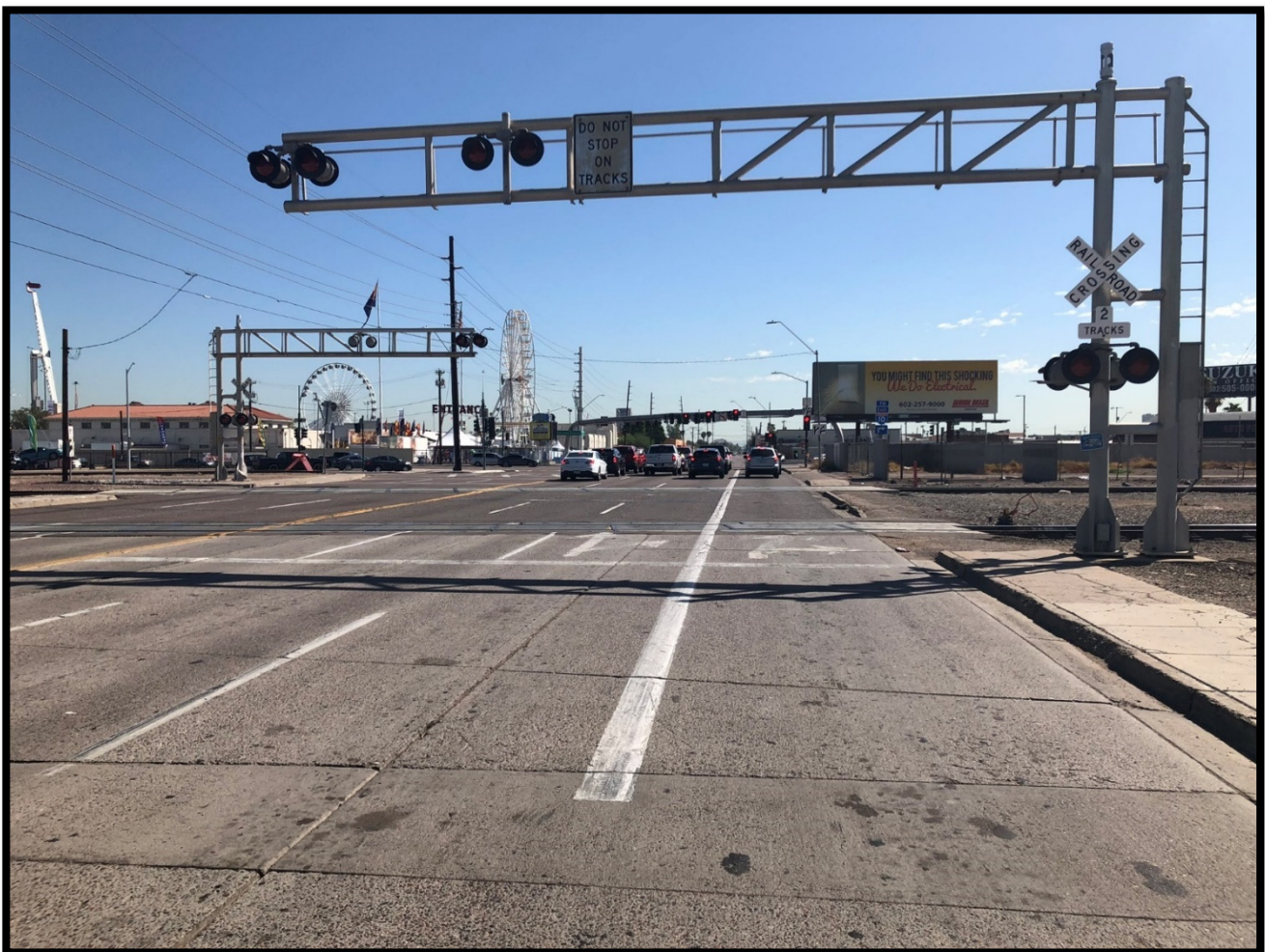
Figure 7 – Railroad Warning Devices at McDowell Road (looking east)
