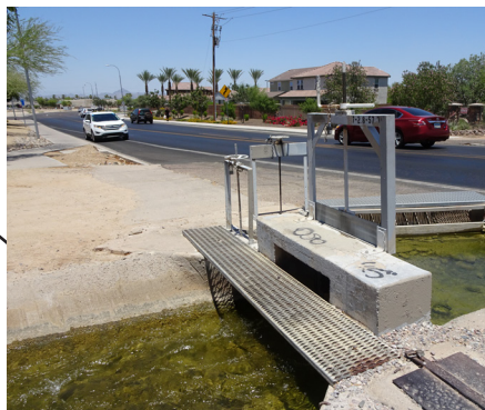
Lack of sidewalk over Highline Canal
