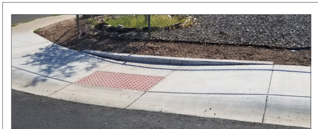
Construction crews are installing hundreds of ADA curb ramps throughout the city, eliminating barriers to mobility for people with disabilities.
