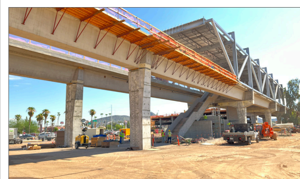
Construction is well underway on the elevated station for the Northwest Extension Phase II
