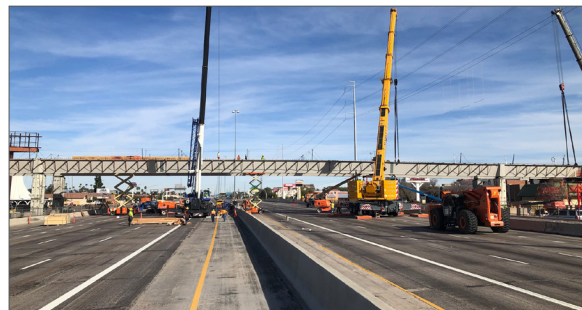
In March of this year construction crews completed bridge girder installation crossing over Interstate 17 for the Northwest Extension, Phase II.
