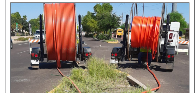
Integration of new fiber optic lines to assist traffic safety and operations.
