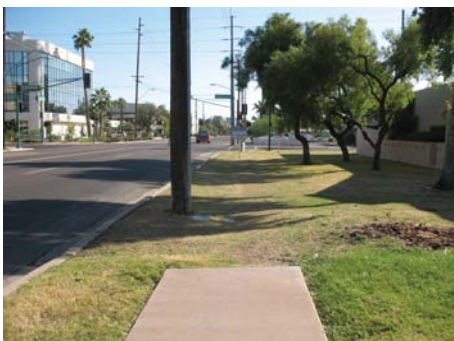
Photo: View south, sidewalk gap north of Virginia
