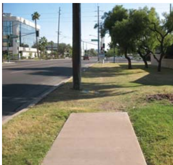
Photo: View South Towards Virginia Avenue Gap in Sidewalk
