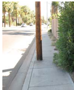
Photo: Existing utilities limit clear footpath width
