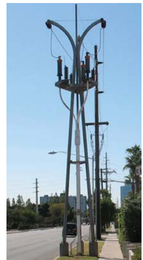
Photo: Utilities obstructions
