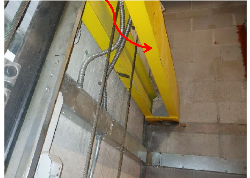
Picture 2: The same "dead" side that holds the side of the cables that do not move. This beam installed by the elevator manufacturer is supported by the hoistway wall. It is doubted this load was communicated to the building designer. This hoistway consists of both masonry and concrete walls.
