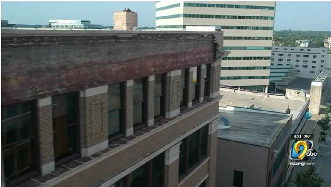
Part of Cedar Rapids building falls to the ground, damages vehicle
