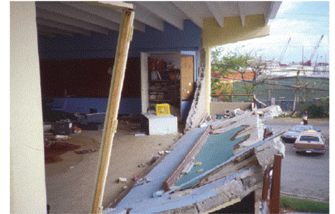
Figure H-13 Collapsed unreinforced masonry classroom wall in the U.S. Virgin Islands during Hurricane Marilyn in 1995 (FEMA, 2010a).
