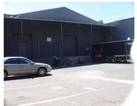
Below: Warehouse building on Jackson street. This warehouse building has the same type of back-in loading docks facing the street.
