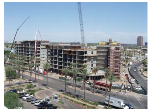
Alta Phx project under construction at 5th Street & Fillmore Street. High density development closer to the Business Core
