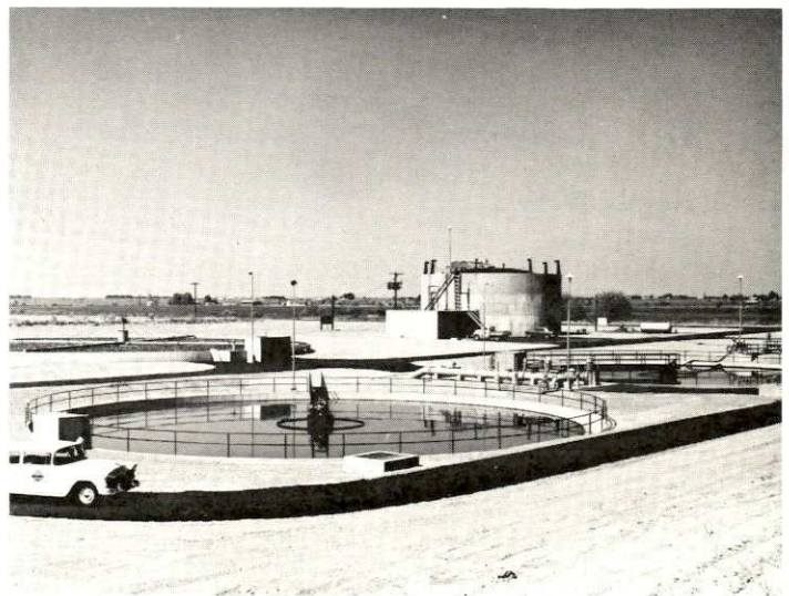
Sewer treatment plant
