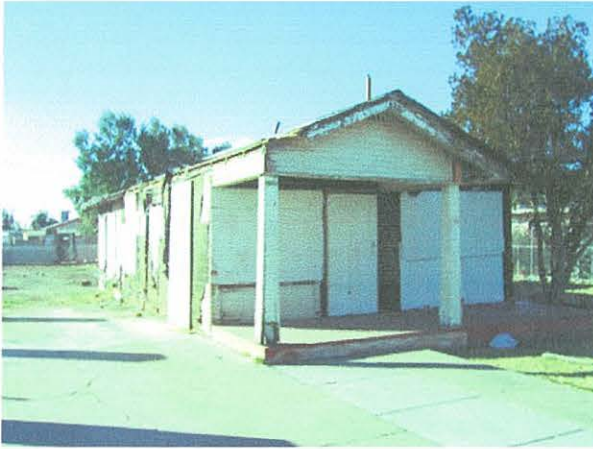
1708 S. 14 th St. General deterioration of a frame bungalow
