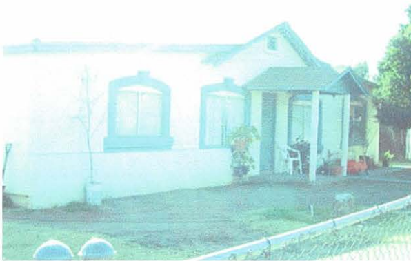
1309 E. Mohave Street Inappropriate additions and alterations to original gable-front vernacular house.
