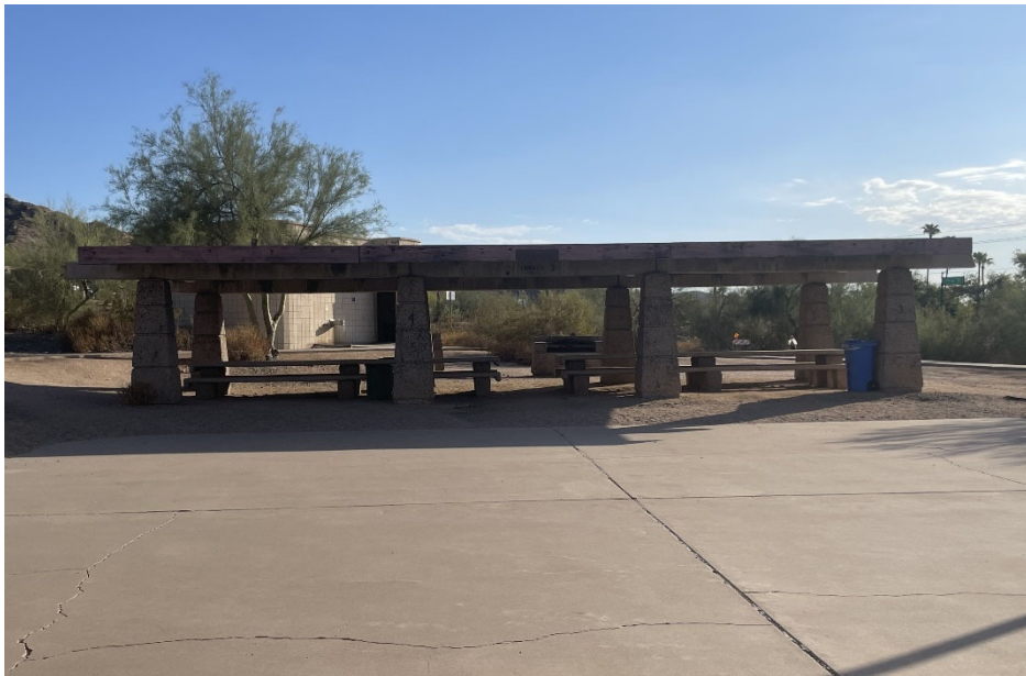
Figure 2. Overview of Building 3A and the concrete event slab. A modern restroom facility is to the rear. View facing north.
