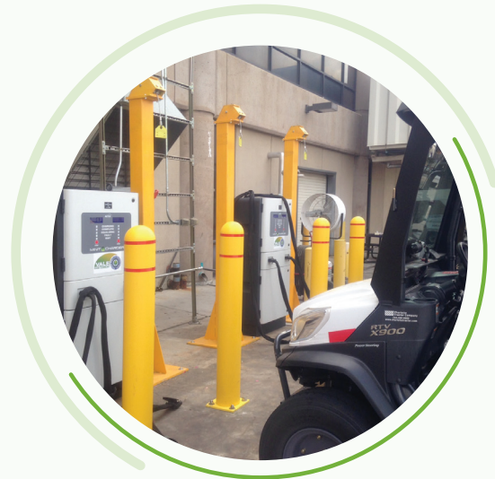
Electric Ground Service Equipment and Charging Stations
