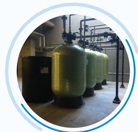
Cooling tower and associated water-pretreatment equipment located at Phoenix Sky Harbor International Airport.
