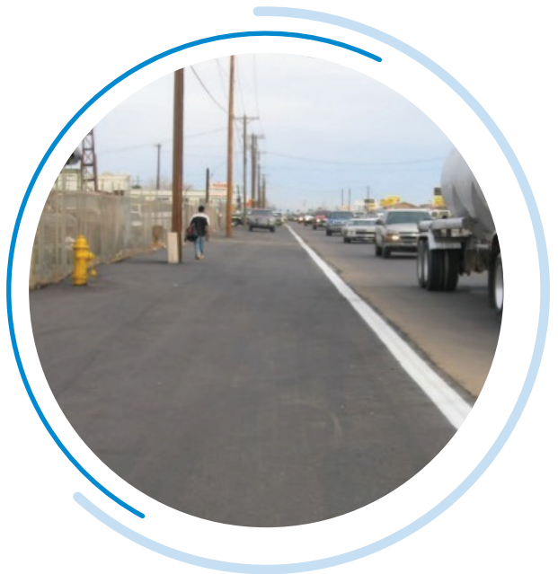
Before and after of surface stabilization on the shoulders of Broadway Avenue.
