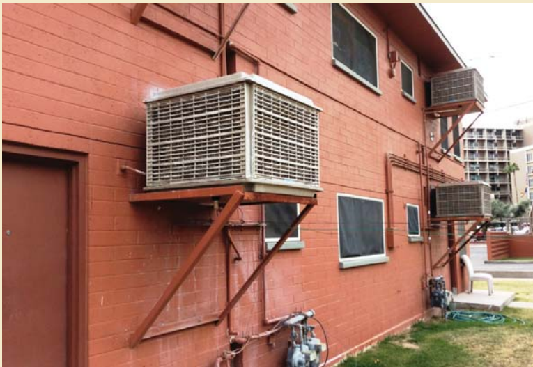
Evaporative cooling units, a.k.a. "swamp coolers"
