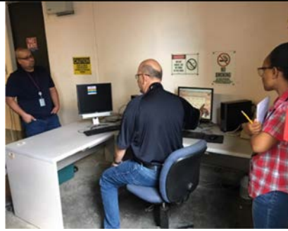
Blower Building Control Room
